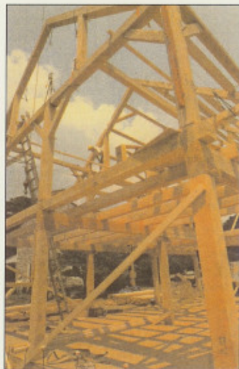
An old-fashioned barn raising occurred several months ago as the beginning of a bank barn to match an existing replica farmhouse.
